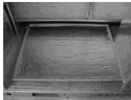
Figure 16: Return down flow plenum with panel
