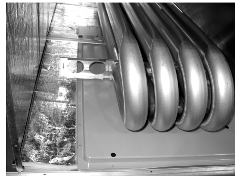
Figure 17: Discharge panel in place
